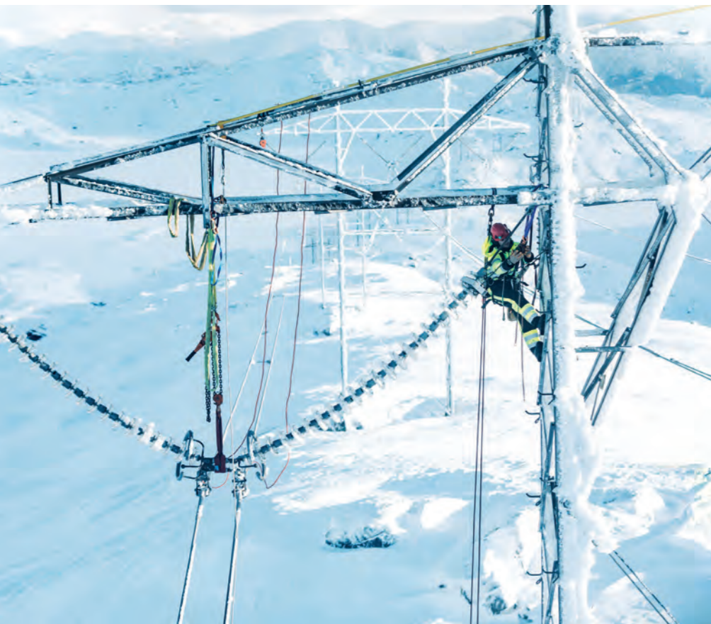
The new sensors that are being installed will send data on the weight of the high-voltage line and when they have to be de-iced, directly via the 4G network.
